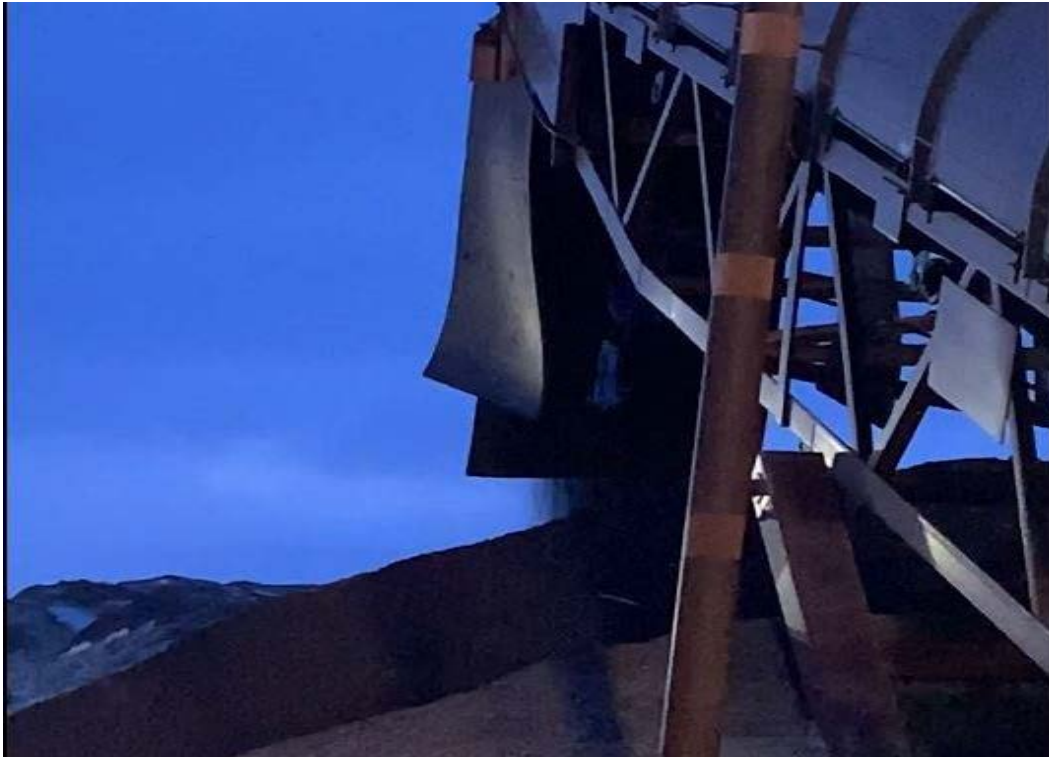
Photo 7-4. Stacker C at the crusher ore stockpile with treated ore.
